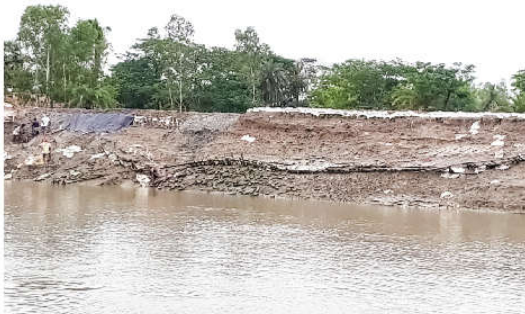
Figure 11. Embankments damaged in West Bengal's coastal areas due to cyclone Yaas.
