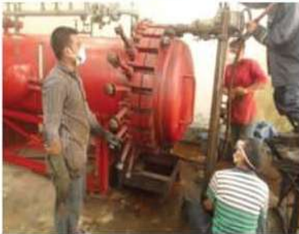
Application of chemicals through pressure treatment plant
